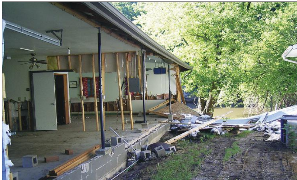
Figure 2-10. Water moving at high velocity destroyed the wall of this home and caused the building to shift on its foundation.
