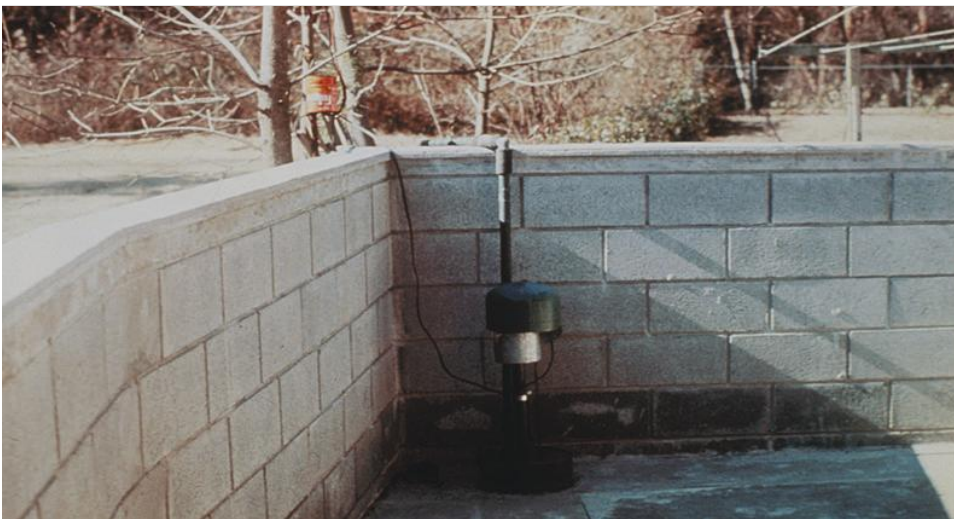
Figure 8-6. Small patio floodwall with sump pump.
