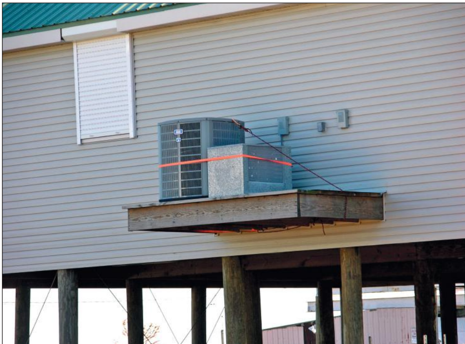
Figure 9-2. Air conditioning/ heat pump compressor mounted on a cantilevered platform attached to a home elevated on an open foundation. (Source: FEMA P-55 Figure 12-2)
