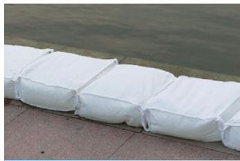
Place First Row of Bags Down, With the Long Side Parallel to Water
