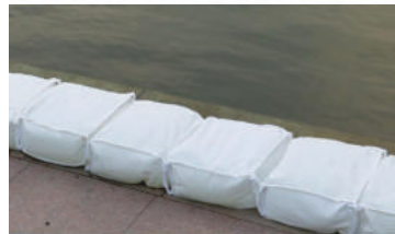
Place a First Row of Bags Down, With the Long Side Parallel to Water
